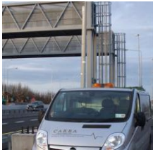
M50 barrier-free tolling systems maintenance
