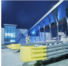
Toll installations & maintenance
